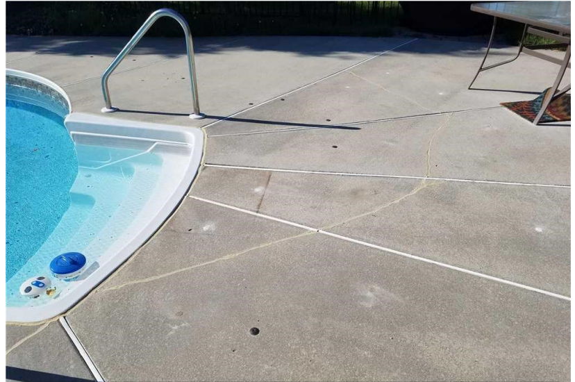
Pictured: a pool decking repair completed by DryZone using Poly-Level® with the cracks sealed with silicone.
